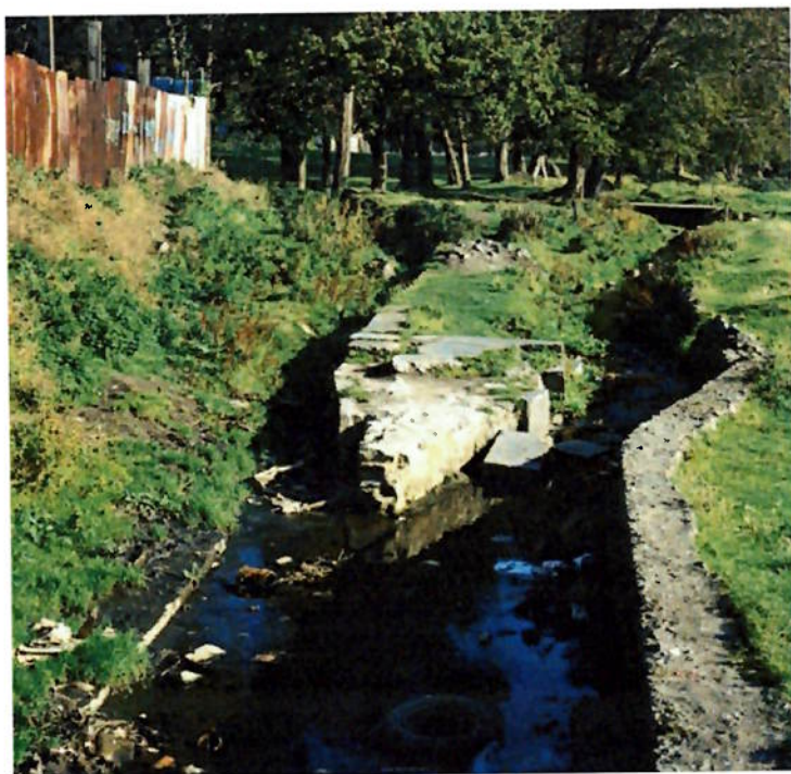
Figure 2. The Tongue in 1977, pre reconstruction. It is unknown if historic fabric survives in the core of the current structure.
