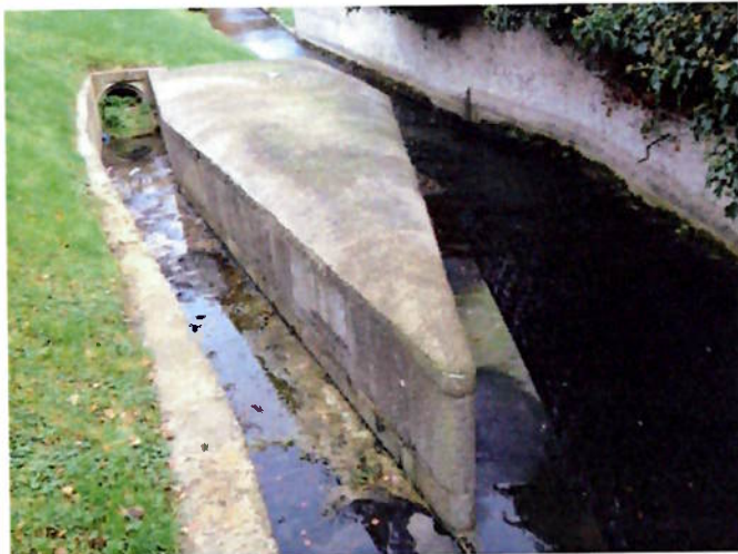
Figure 1. The current appearance of the 'Tongue'. An inscription on the north face states "STONE BOAT/BUILT 1245 A.D./RESTORED BY/TIERNAN BUILDERS/1990 A.D."
